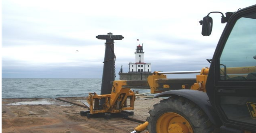
The crane leaving the lighthouse deck for the first time since it was installed in 1931.
